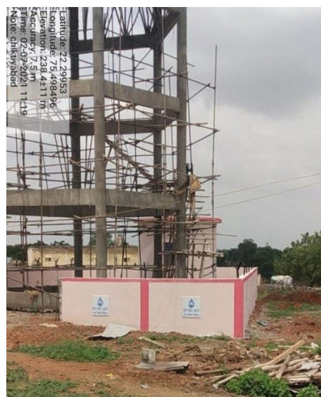
Overhead tank and sump tank under construction in Chilur village in MP
