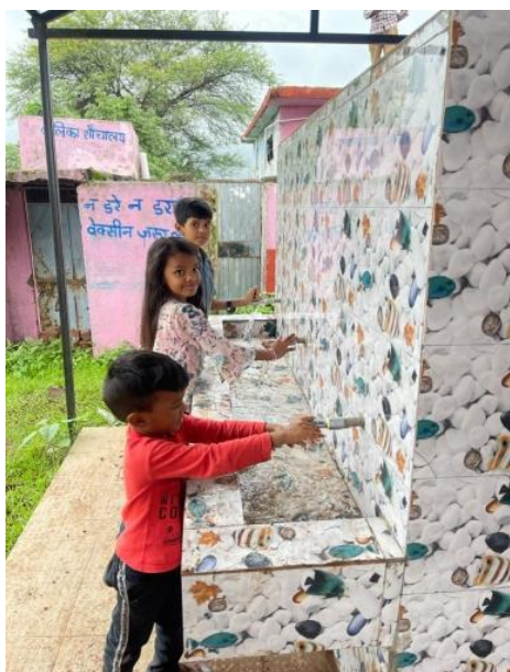
Tap connection provided under the 100 days campaign in a rural school in MP
